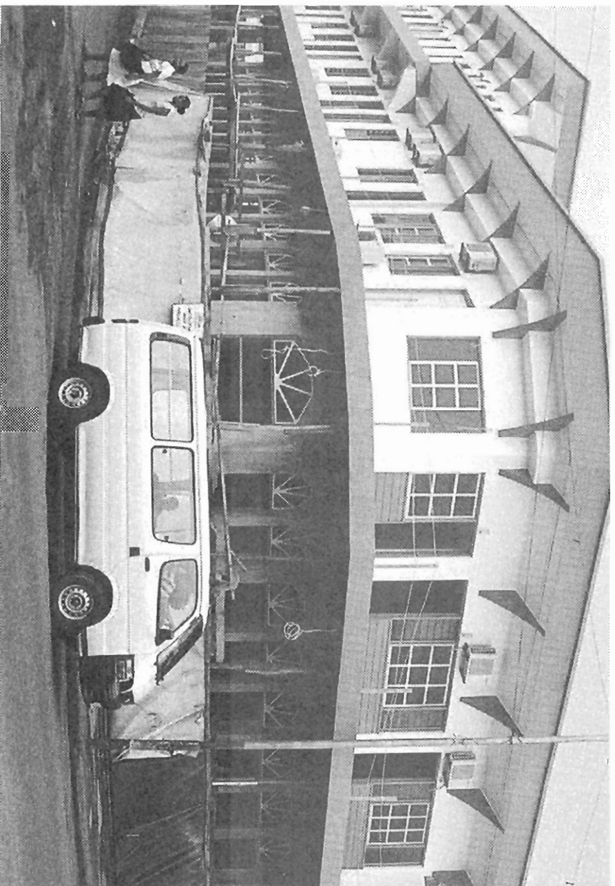
The construction site of a new hotel at the heart of Labasa town. Photo: KHAILASH RAO
